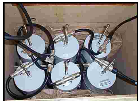
New GARA duplexers installed for the 145.150 machine
